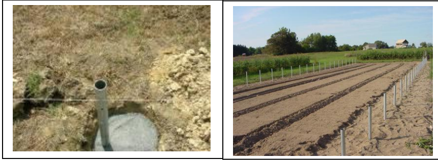
Figure 7. Corner posts can be set in cement to provide strength for the high tunnel structure. A leveling line is used to ensure each ground post is level. (Photo credit: A. Montri)
